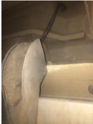
Figure 28: Winch Wires from Bottom Side
