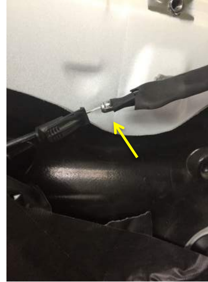
Figure 54: Strap Fork with Loose Heat Shrink
